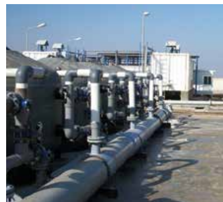
▲ Each plant consisted of 10 x Micron SMD2000 Filters.
