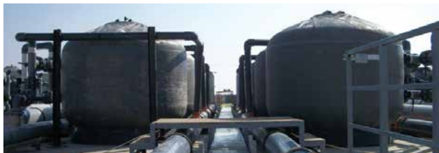
▼ Combined prefiltration for the 4 plants is approximately 1000 - 1100 m 3 /hr.
